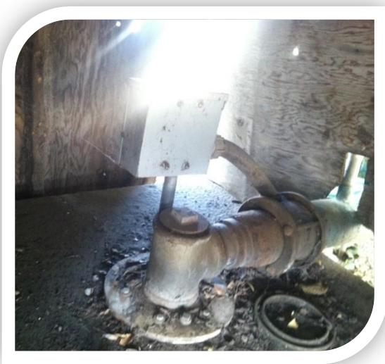
Above: An active 12-in steel casing irrigation water supply well constructed in 1980.
